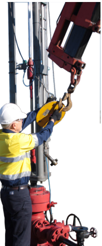
"Rigging up" to lift well head section is done from ground level
